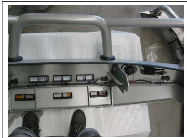
Figure 8: Secure wiring into rear of bar. NOTE: Parking sensor wiring loom shown.
